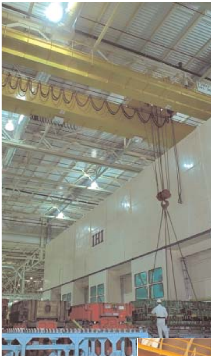
30t Press Shop Crane Honda (UK)
