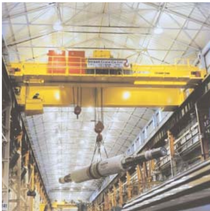
130t Turbine Handling Crane G.E.C. Alsthom
