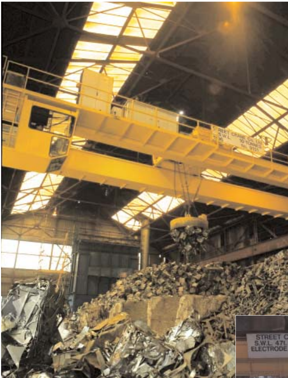
10t Magnet Scrap Handling Crane George Fischer Foundry
