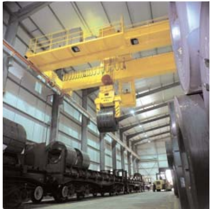
35t Coil Handling Crane E.W.S. Limited
